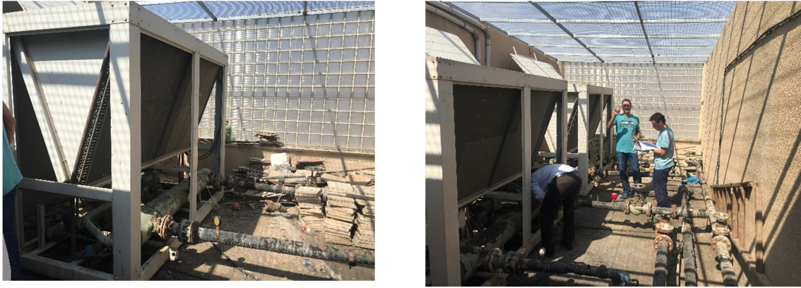
Picture 7: Existing chillers on the roof of the building
