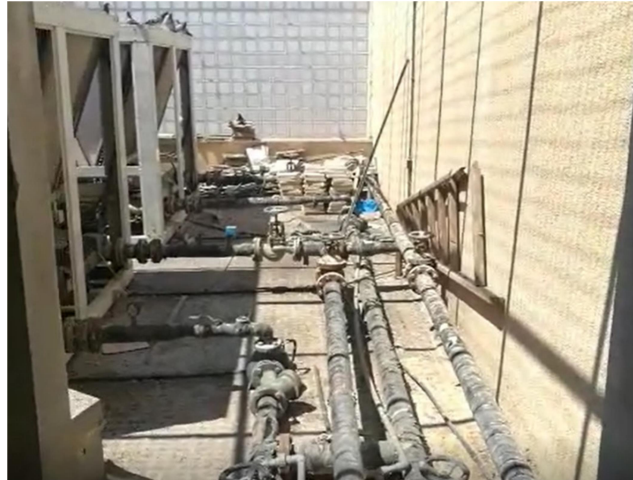
Picture 14: Existing water distribution network of the two installed chillers
