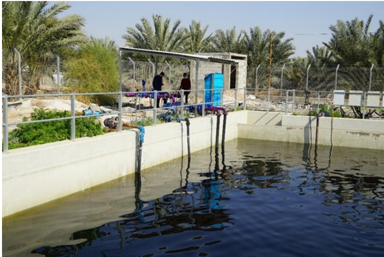
Fig. 10 The "irrigation tank" at the WWTP of Jericho. Pipelines and pumps of the single farmers who buy this water are shown. The pipeline of the MEDISS project is visible as well, under the roof
