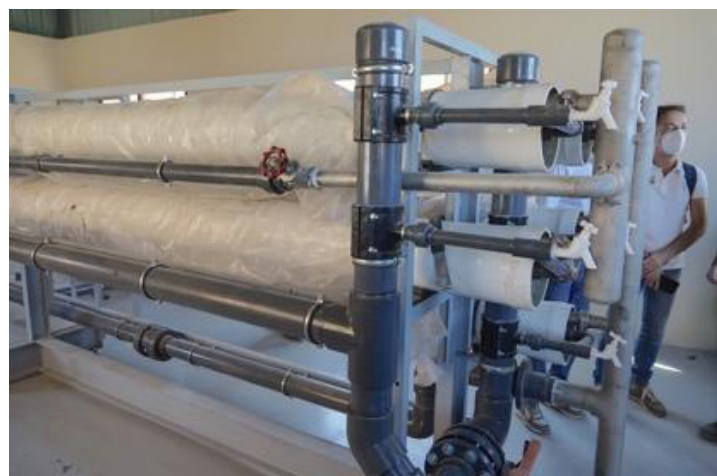
Fig.1 One component of the new desalination plant set up in Al-Risha by the AWC
