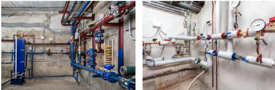
Figure 11: Individual automatic heat point with weather compensation control
