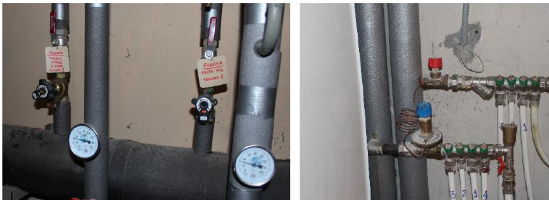
Figure 14: Balancing valves for HVAC systems
