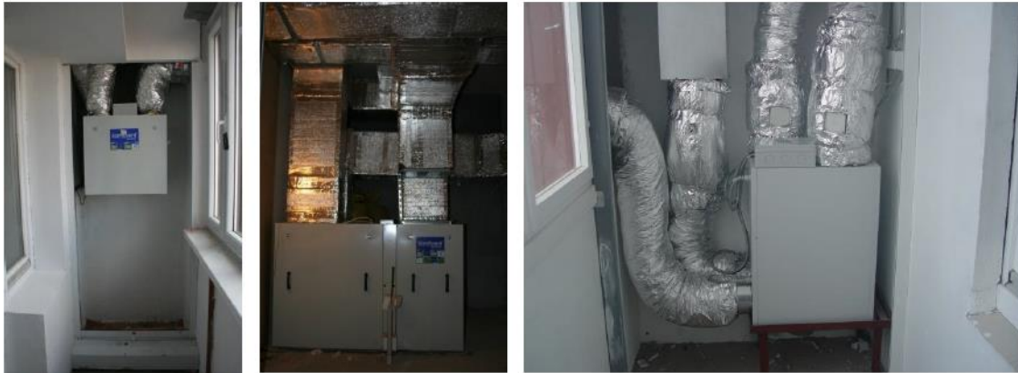
Figure 16: Heat recovery unit for mechanical inlet and outlet ventilation
