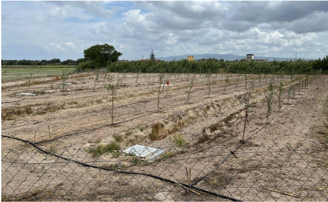
Figure 35. Emergency irrigation system by drip irrigation
