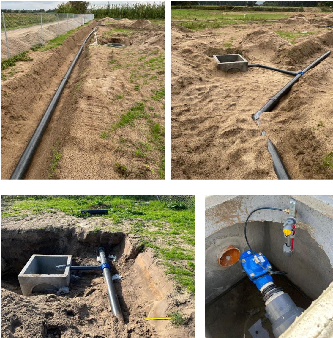
Figure 30. Buried pipelines and connection with the pits (upper panels) and details of the floating valves in the pit (lower panel).
