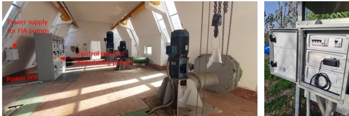
Figure 27. Panel for the FIA supply power installed in the facility of the Luri dewatering pumping station (left) and auxiliary power panel for controlling the pumps from the FIA field.
