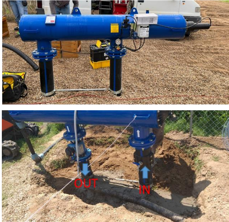
Figure 29. Filtration system installed in the field
