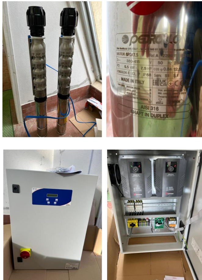
Figure 28. Pumps (upper panels) and Inverter (bottom panels)
