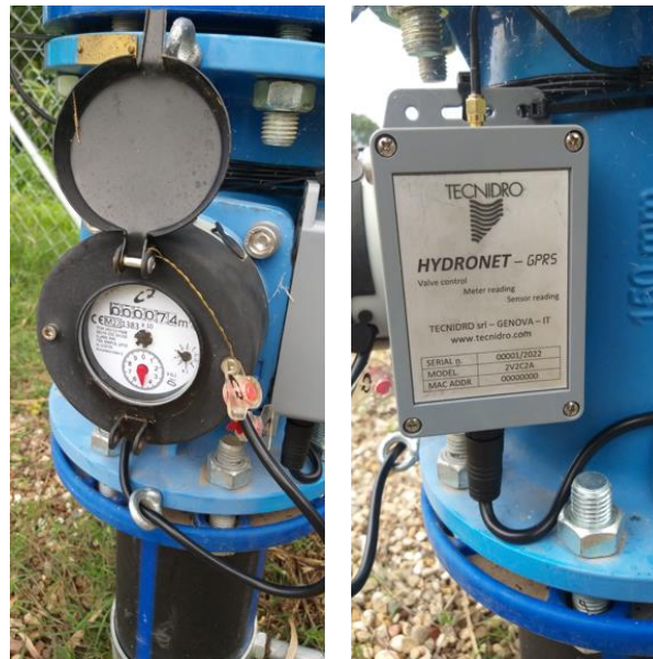
Figure 38. Analogic flow-meter and GPRS device for remote transmission of the flow rate data
