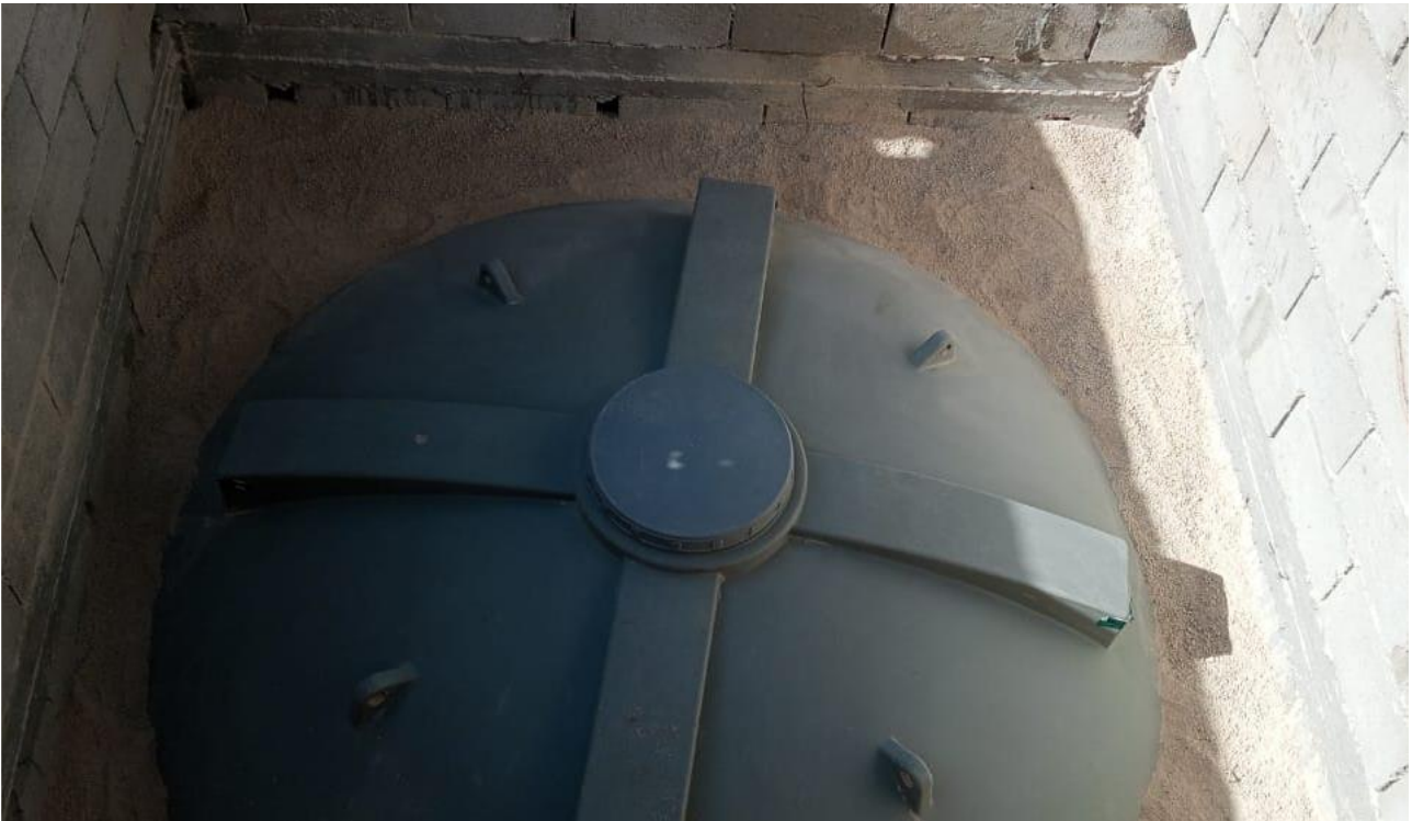
Figure 47. Regulation tank for the solar system.
