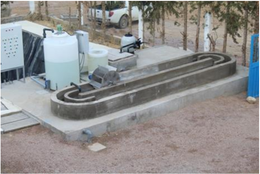
Figure 63. Solar raceway pond reactor
