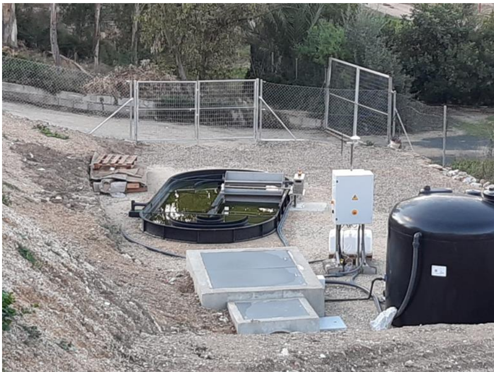
Figure 18. The completely installed solar raceway pond reactor and auxiliary systems.
