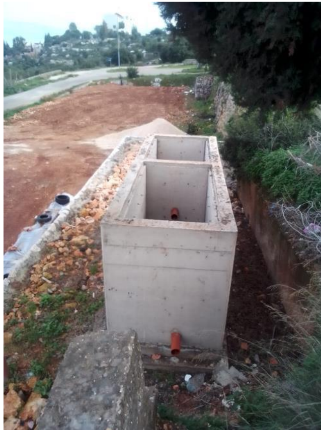
Figure 43. Detail of the tank for the pretreatment elements.
