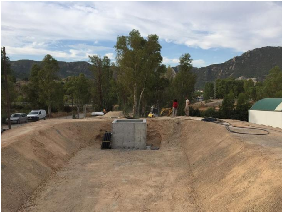
Figure 9. Water drainage collection box.
