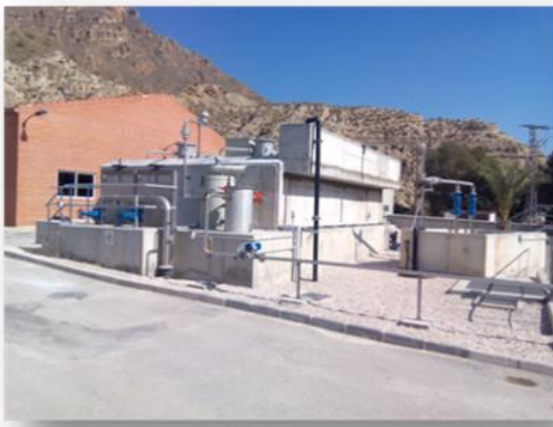
Figure 4. The anaerobic reactor.
