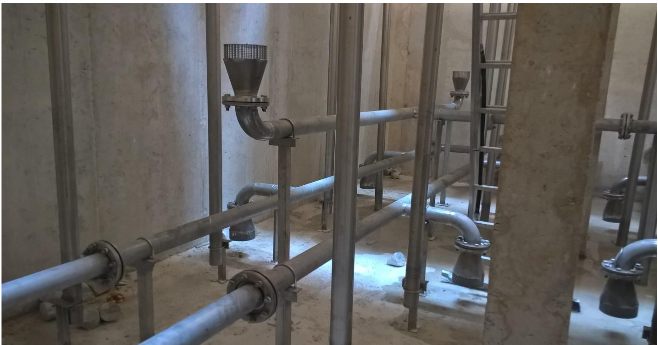
Photo 2 Inner of the UASB reactor.
