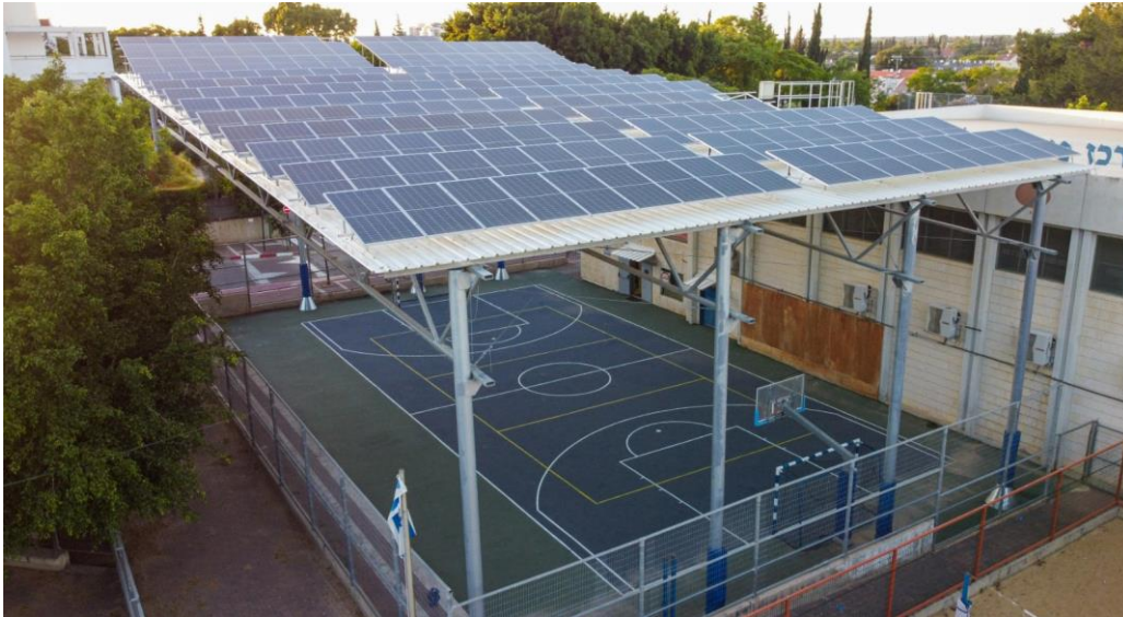
Figure 6: Innovative use of sports ground for the production of solar-based electricity, providing a win-win solution with revenue for the municipality, safe sun-shielding for the comfort of basketball players, increased energy independence and decrease of CO2 emissions and air pollution in Kfar Saba.
